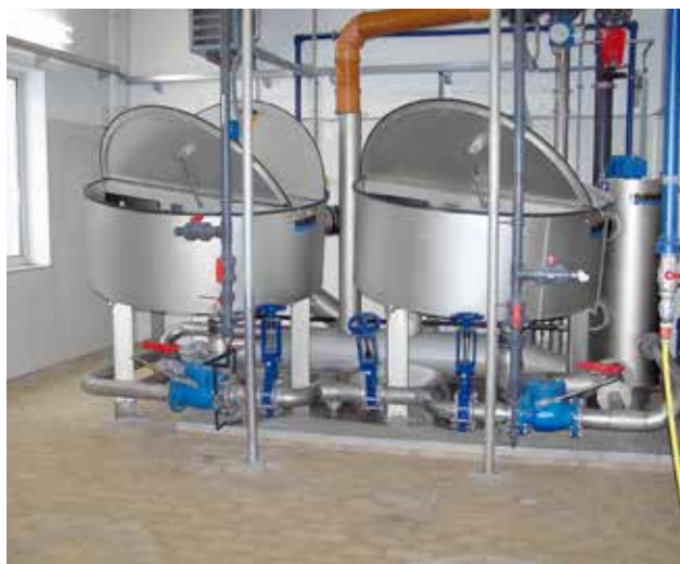
Zwilling-Installation in engem Raum.
