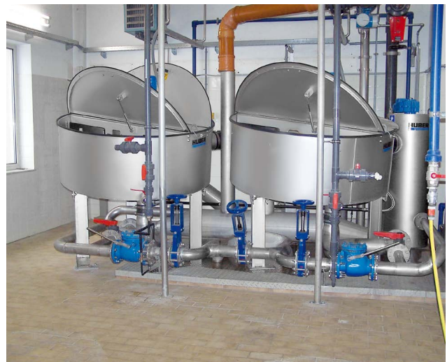
Zwillings-Installation in engem Raum.
