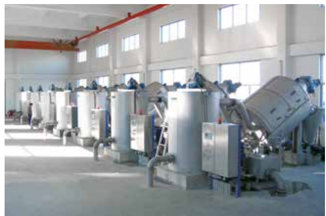
Eight screw thickeners handling 600 m 3 /h.
