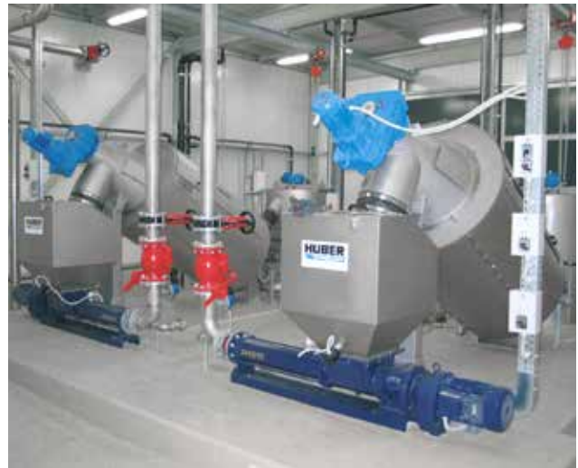
Two HUBER Rotary Screw Thickener S-DRUM units for 80 m 3 /h.
