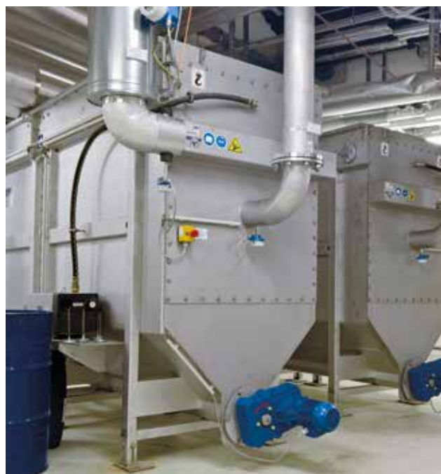
Municipal wastewater; 2x RoWin size 8; heat extraction capacity 560 kW heating / 1,000 kW cooling.
