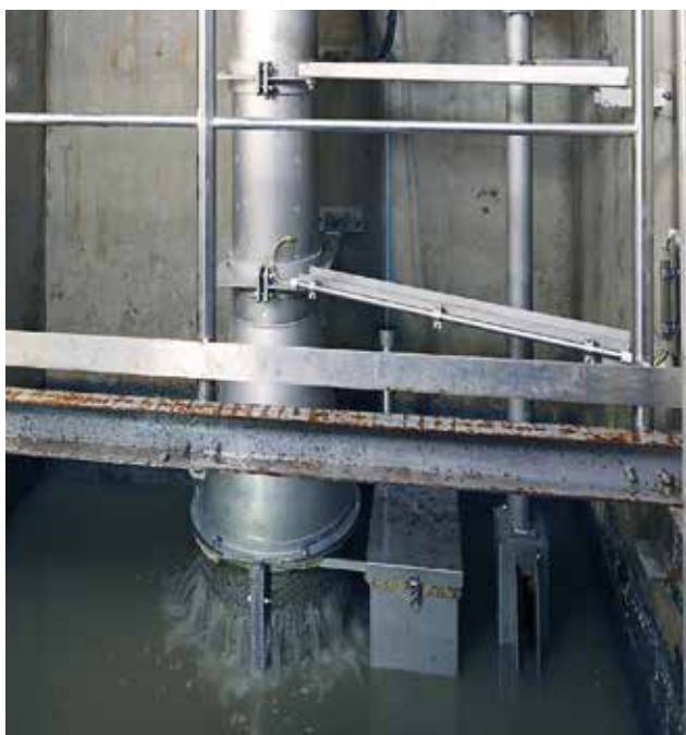
Wastewater pre-screening in the intake structure with a HUBER Pumping Stations Screen ROTAMAT® RoK4.
