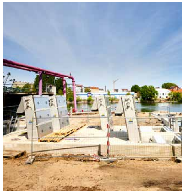
Installation of the HUBER Multi-Rake Bar Screen RakeMax® in Berlin-Schöneeweide (source: BTB).
