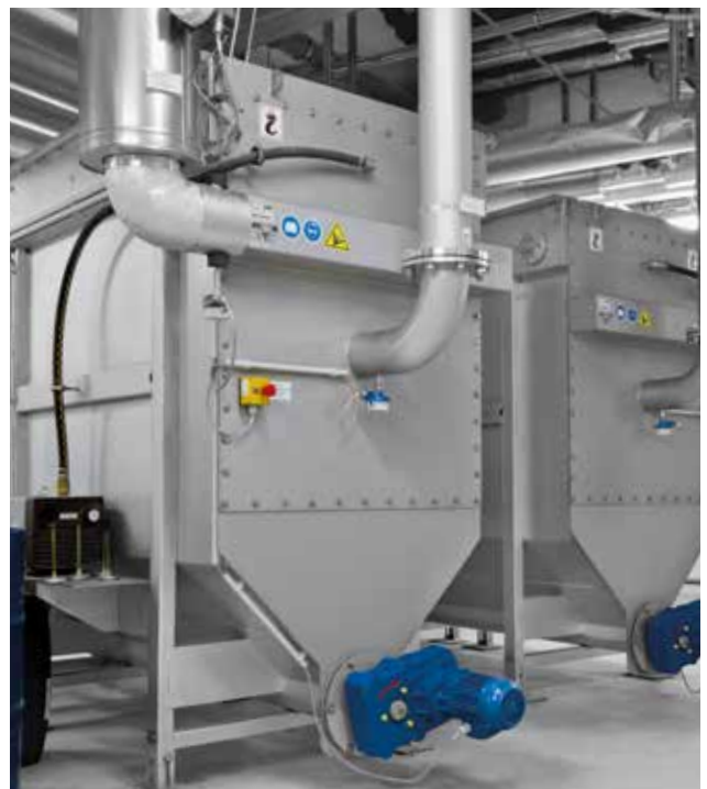
Two HUBER Heat Exchangers RoWin installed in parallel in the tank.
