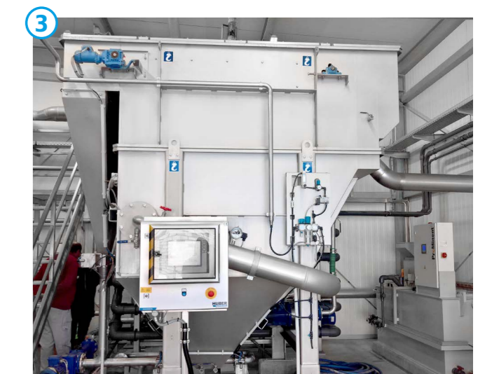
HUBER Dissolved Air Flotation Plant HDF.
