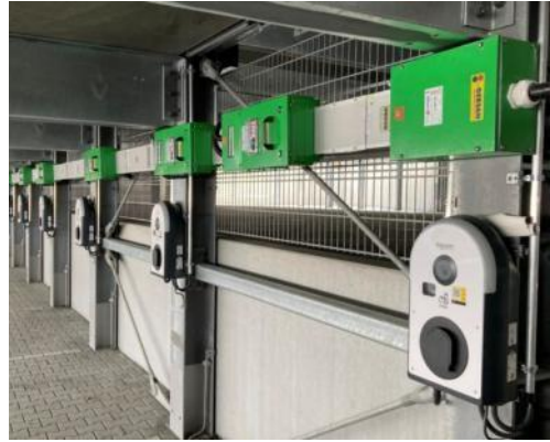
Fig. 46: State-of-the-art charging stations for employees' electric cars and company cars.
