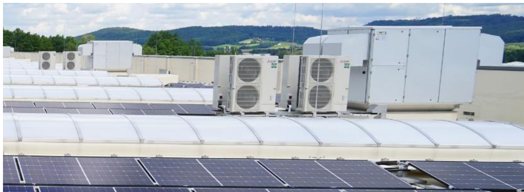
Fig. 19: Ventilation systems with heat recovery and heat pumps installed on the roof of the production hall.
