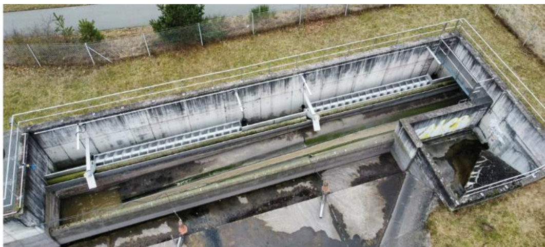
Fig. 33: A discharge structure with HUBER Storm Screen ROTAMAT® RoK1 TS units that operate reliably even in heavy rain, combined with large amounts of screenings.
