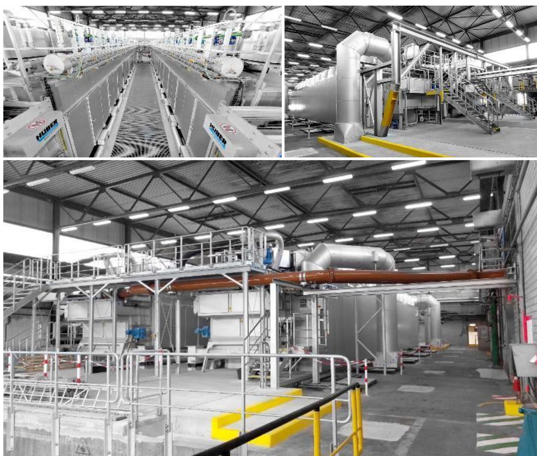
Fig. 51: HUBER Belt Dryer BT installed at BASF in Ludwigshafen. Since 2023, 90,000 tonnes of dewatered sludge have been dried from 27% to 45% dry residue (DR). This saves coal as a supporting fuel for sewage sludge incineration and avoids more than 24,000 tonnes of CO 2 emissions.
