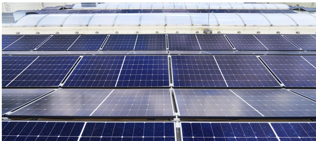
Fig. 18: The solar panels installed on the roofs of the production halls have a total output of 1122 kWp.
