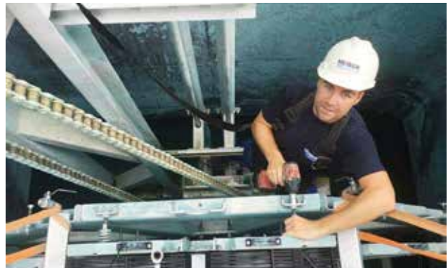
Successful start of operation due to professional installation.
