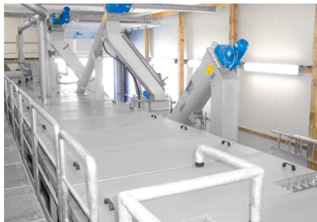
Complete Plant with integrated Grit Washer.
