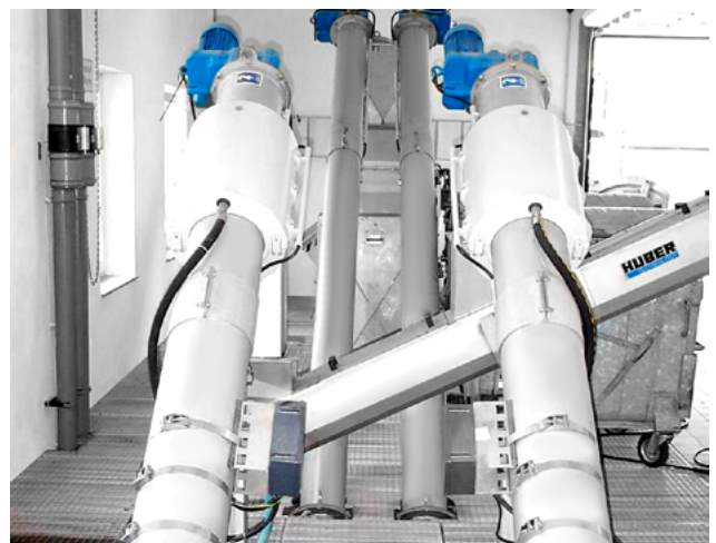
Underground, redundant HUBER Complete Plant ROTAMAT® Ro5.
