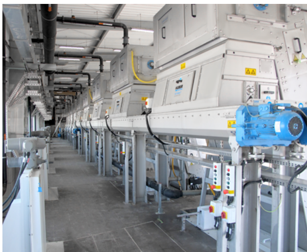
Redundant conveyor using a double trough diverter.
