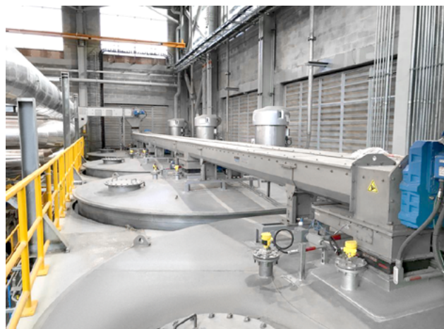
Horizontal transport of dried sewage sludge.
