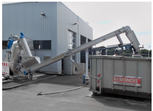
Rotating Screenings Distribution Screw Ro8 TC.
