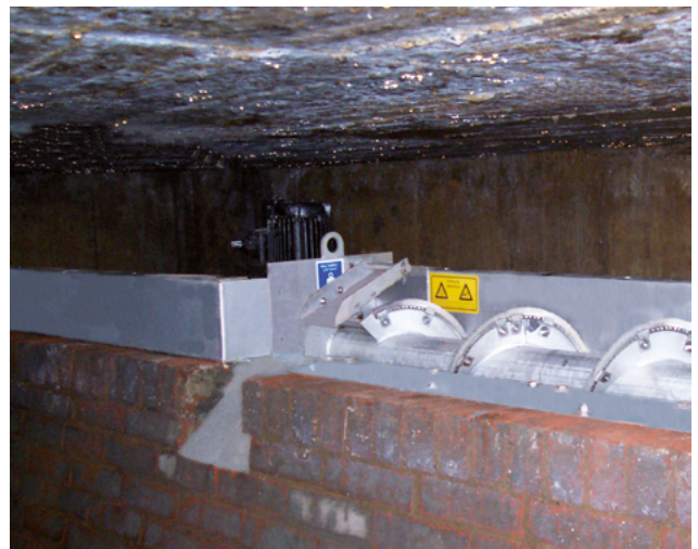
Return of screenings into the sewer.
