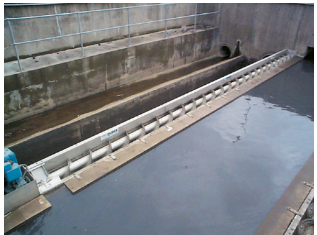
HUBER ROTAMAT® Storm Screen RoK1 installed in a stormwater discharge channel.
