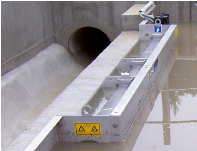
HUBER Storm Screen ROTAMAT® RoK2 before overflow.
