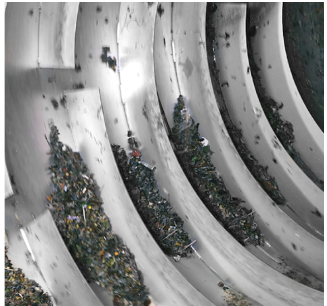
50 l screenings removed per rotation.
