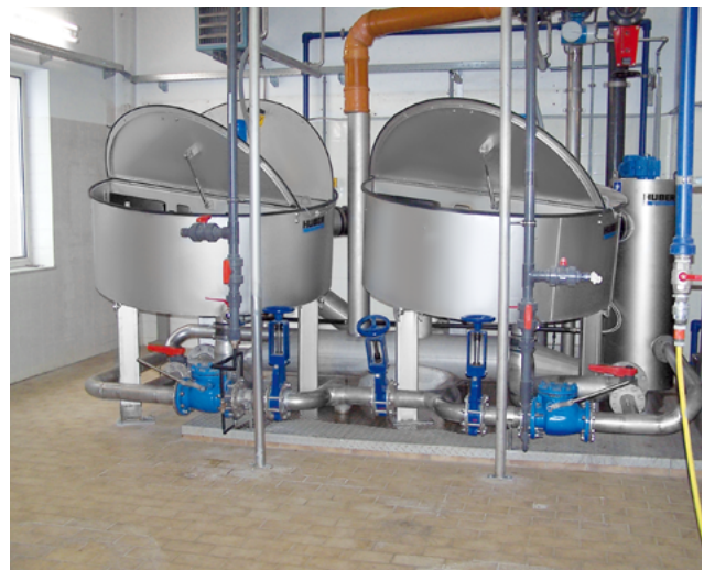
Two units installed in confined space.
