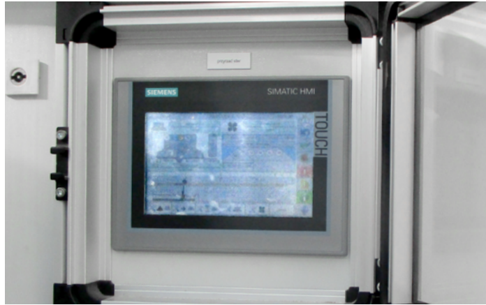
Touch panel for plant control.
