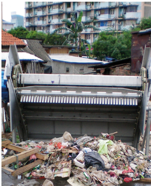
Free discharge of the screenings prevents blockages.
